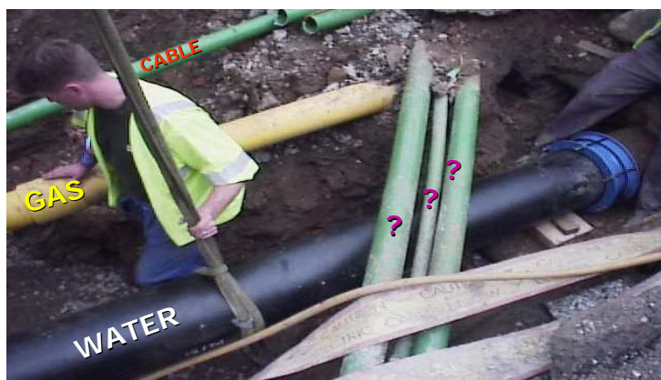
Figure 1: A not unusual feature of modern buried services
