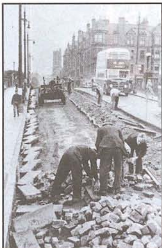
What lies beneath. The historical problem of buried services.
